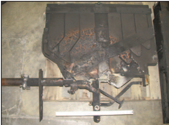
Failed Circuit Breaker Assembly
